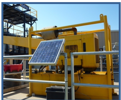
BP330 Charging Crane Battery Bank
